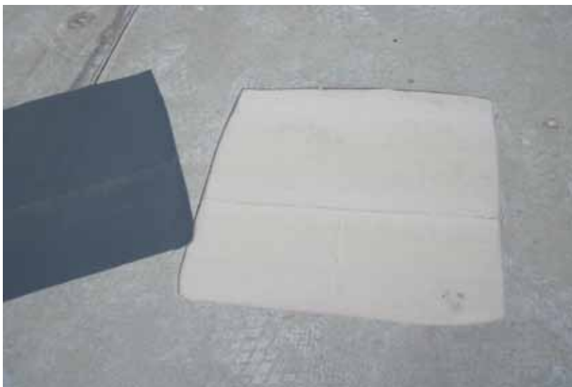
► Photo 1: The membrane and insulation interface at the Target store in Novi, Mich.
