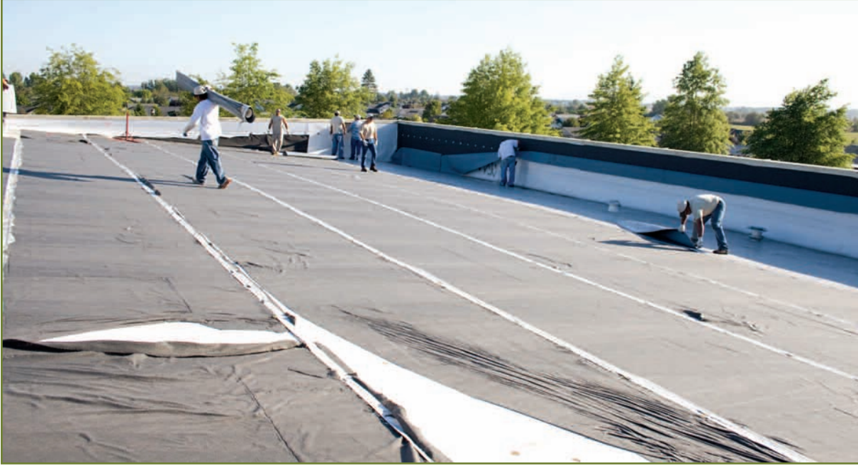
Contractors segregate the fasteners from the seam strips after the main vinyl sheets have been removed from the substrate. Image courtesy Vinyl Roofing Division, CFFA.
